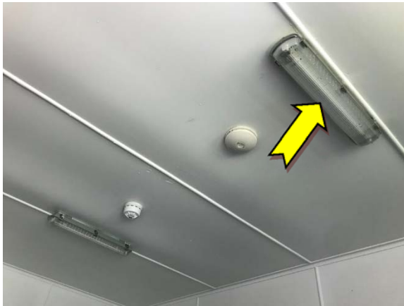
Photo 3. Interior, throughout, single tube fluorescent light fittings – suspected PCB-containing capacitors.
