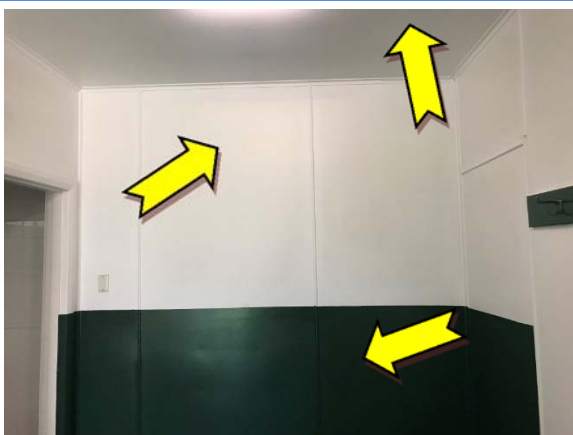
Photo 5. Interior, throughout, walls and ceiling – suspected lead-containing white and green upper coloured paint systems.
