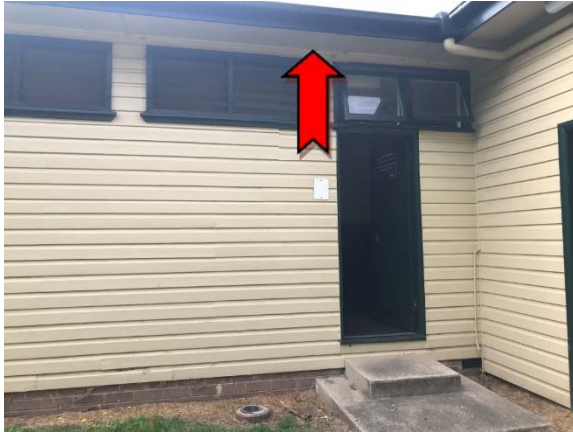
Photo 1. Exterior, throughout, eaves – asbestos-containing fibre cement sheeting.
